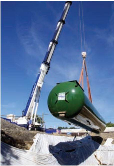
Figure 3 Belowground propane tank installation Photo courtesy of Highland Tank Company
