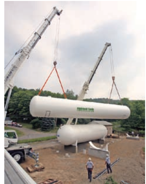
Figure 2 Aboveground propane tank installation Photo courtesy of Highland Tank Company
