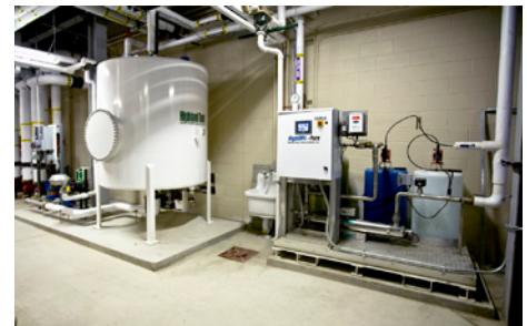
Rainwater Harvesting Systems
