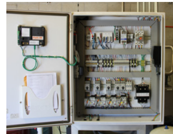
The above images show the front of the control panel with touchscreen and the inside components of the panel.
