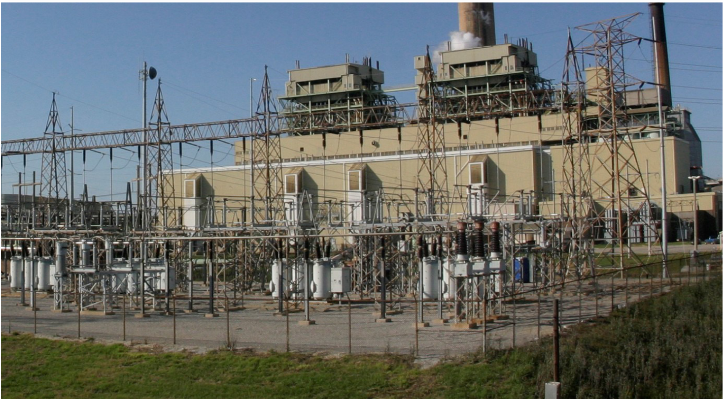
Wastewater storage tanks and oil/water separators may be used as part of an electric power facility drainage system to meet the secondary containment requirements.
