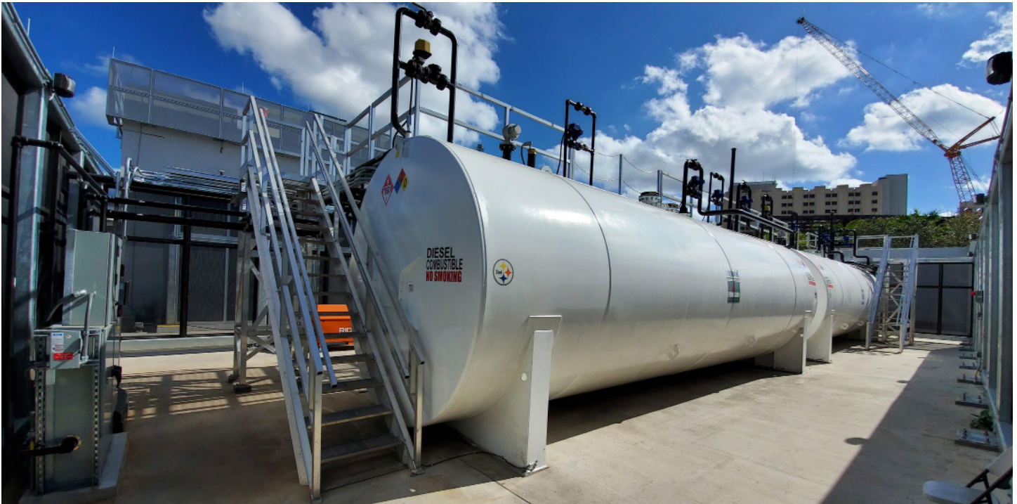
A Fireguard® tank for diesel storage at a Central Energy Plant.
