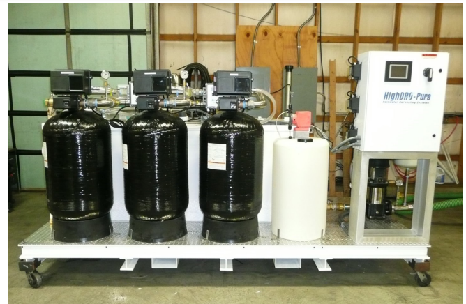
Rainwater Harvesting packaged skid-mounted system .
