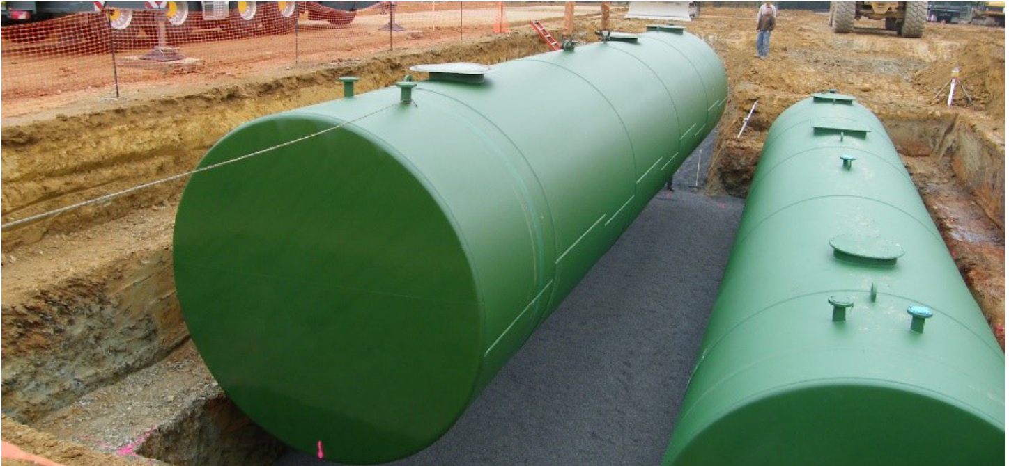
Water collection tanks.
