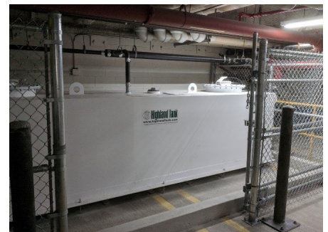
Rectangular Passive Grease Interceptor
