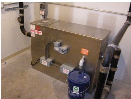
Automatic Grease Interceptor (AGI)
