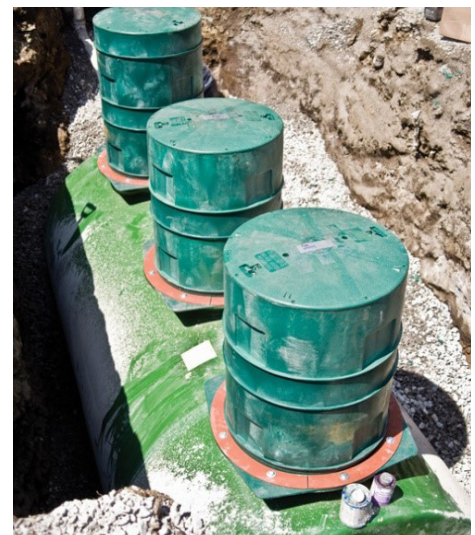
Underground Passive Grease Interceptor
