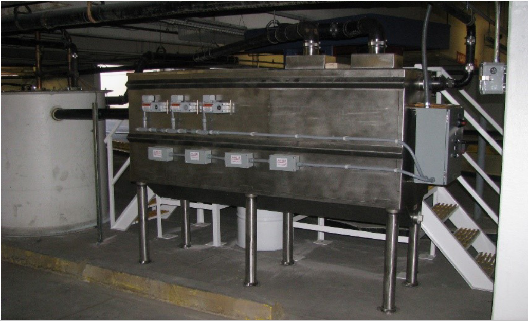
A large volume grease interceptor in a parking garage.
