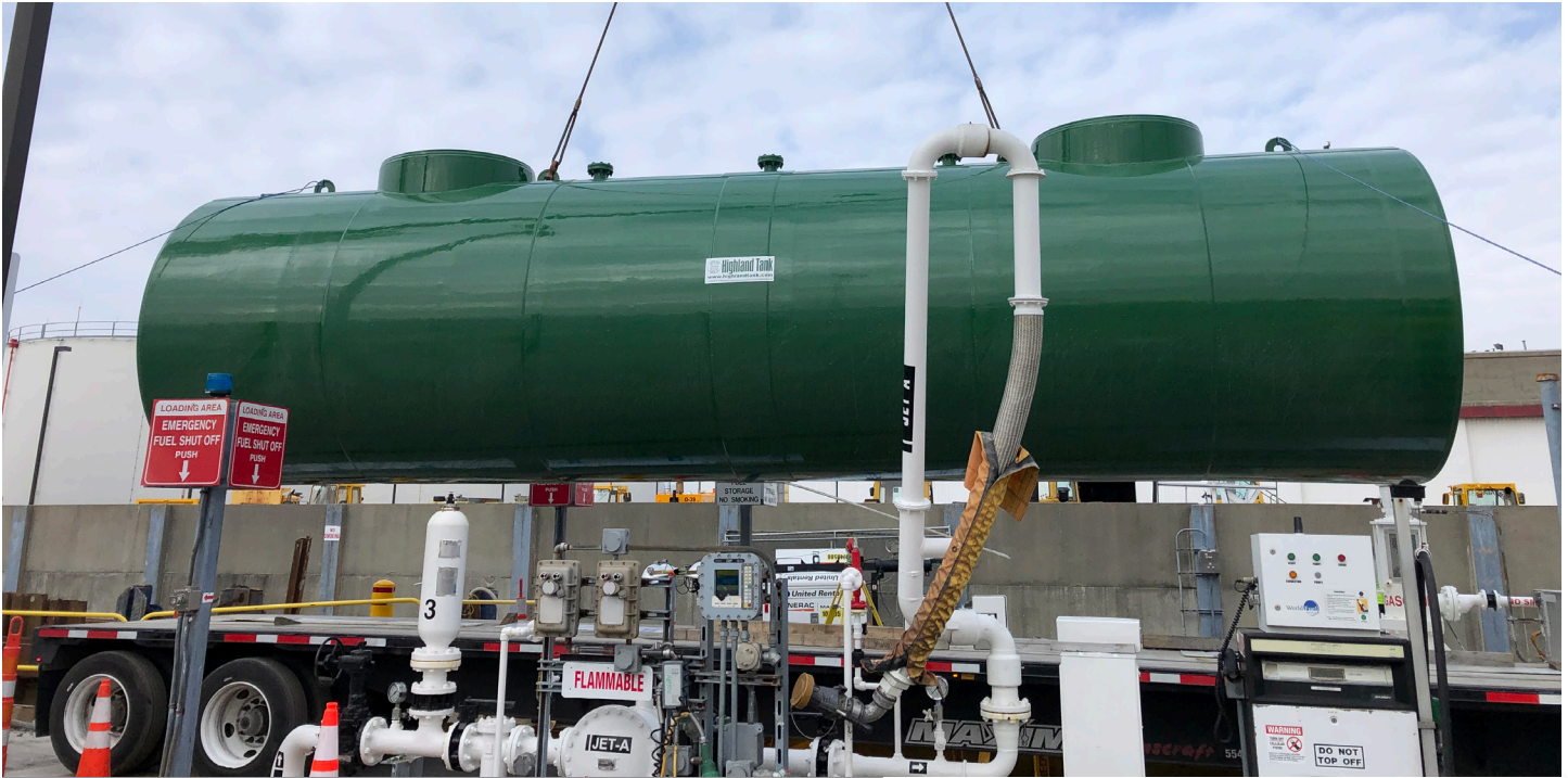
A Highland Tank 20,000 gallon storage tank is installed at an airport.
