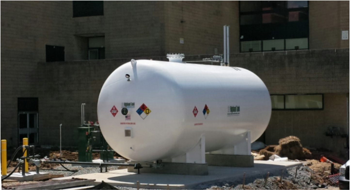
Highland Tank's LPG vessels are designed and constructed to ASME, Section VIII, Division I and NFPA 58 "Liquefied Petroleum Gas Code" for stationary use vessels.
