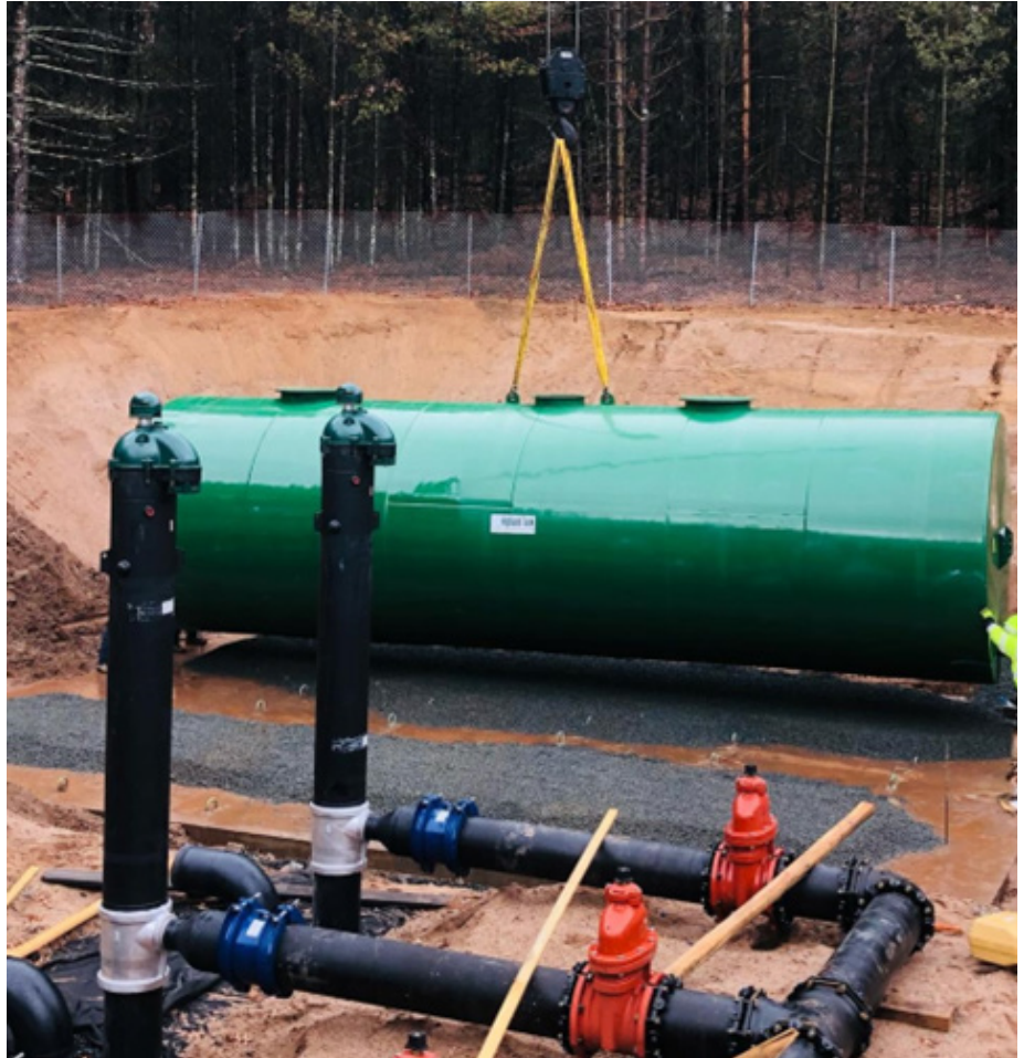
A 20,000 gallon HighGuard bottom Drain Fire Protection System.
