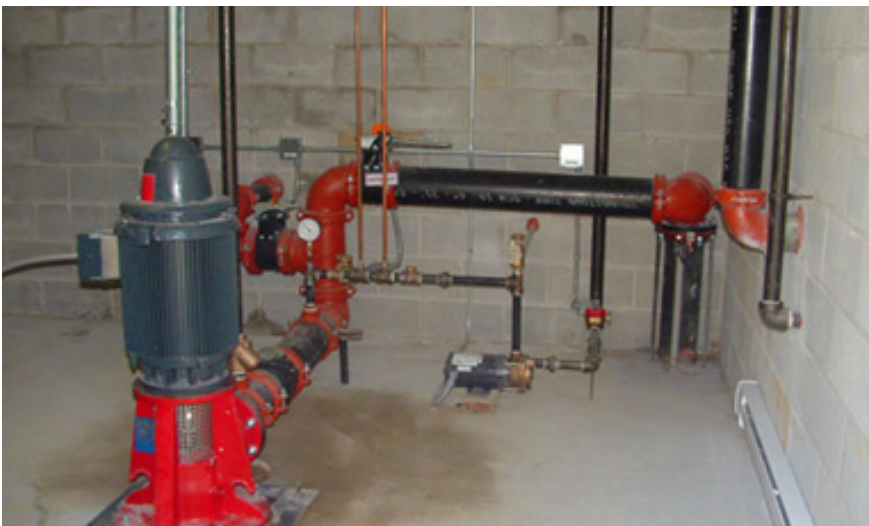
A 20,000 gallon HighGuard fire protection tank with pump well.
