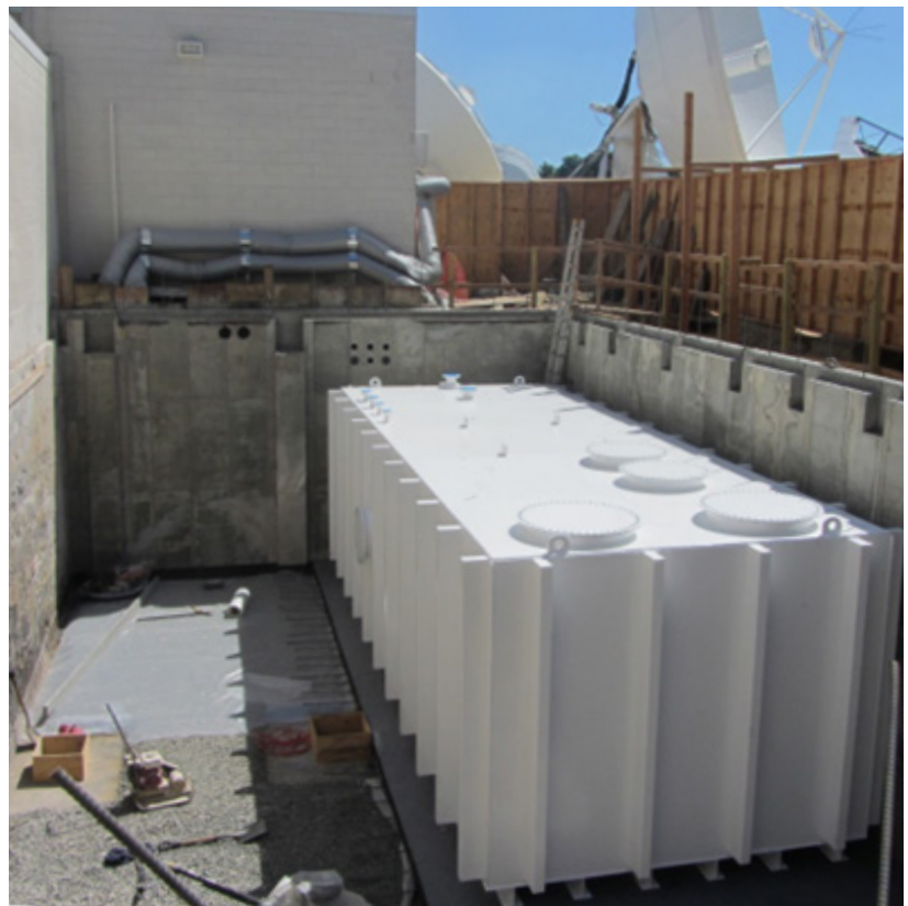
A 15,000 gallon aboveground break tank with external bracing.
