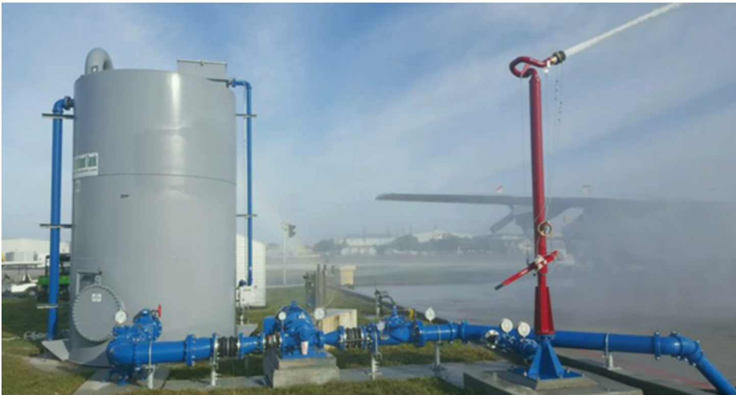
A 10,000 gallon vertical bottom drain fire protection system.
