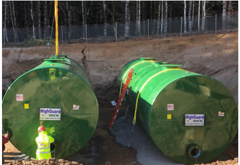
Underground fire protection tanks with HighGuard coating system.
