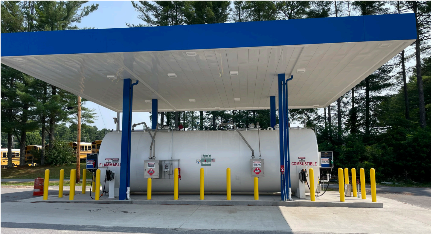
A 20,000 gallon two-compartment Fireguard tank for a school bus depot with High-LINK fuel management system.
