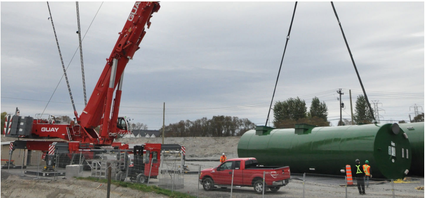
EPA regulations for power plants typically include SPCC plans requiring an oil/water separator
