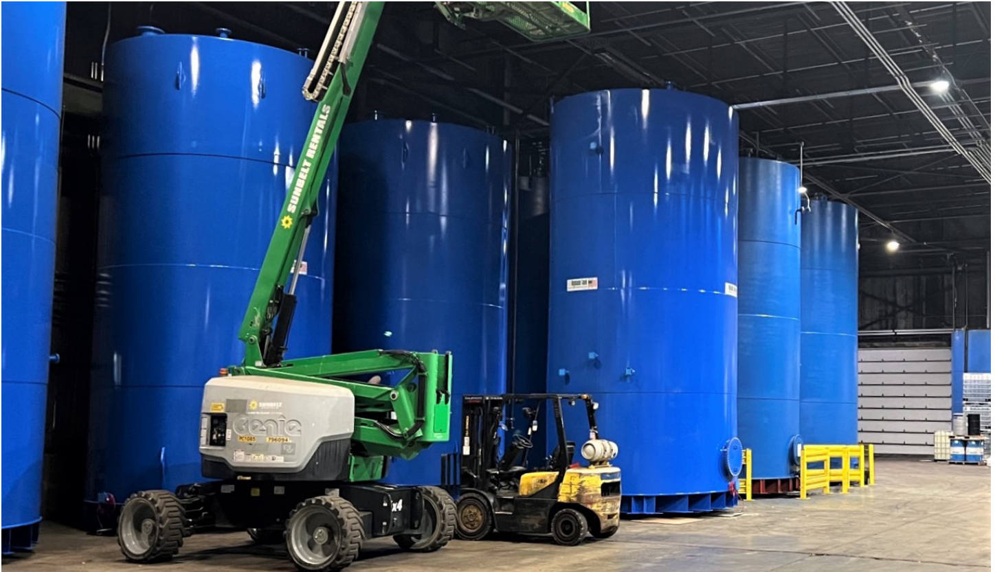
Highland Tank's petroleum storage tanks provide safe and dependable bulk storage for all types of products.
