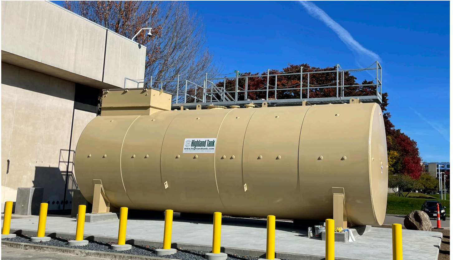
A Highland Tank Fireguard® fuel storage tank at a critical facility.
