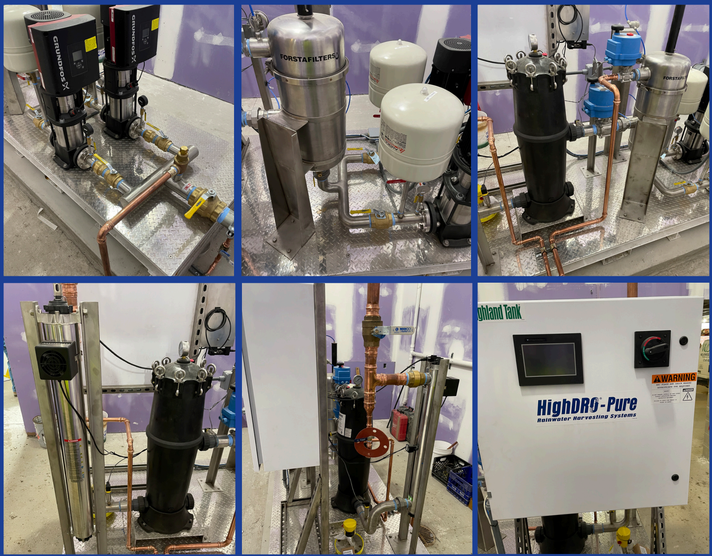
Highland Tank supplied three 30,000 gallon cistern tanks and the rainwater harvesting system show above as part of a stormwater management plan.
