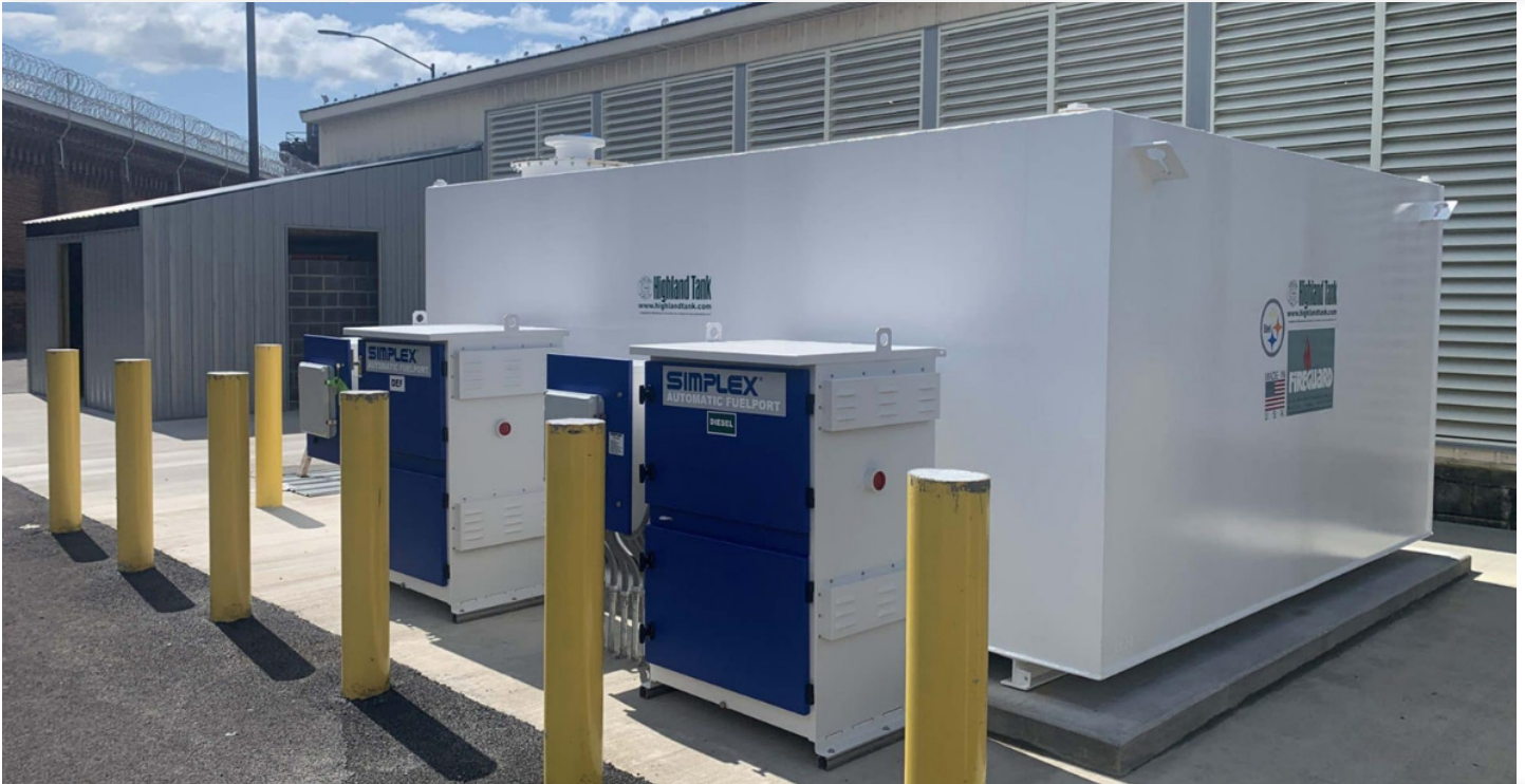
Shown above is a Highland Tank rectangular FIREGUARD® tank with fuel port
