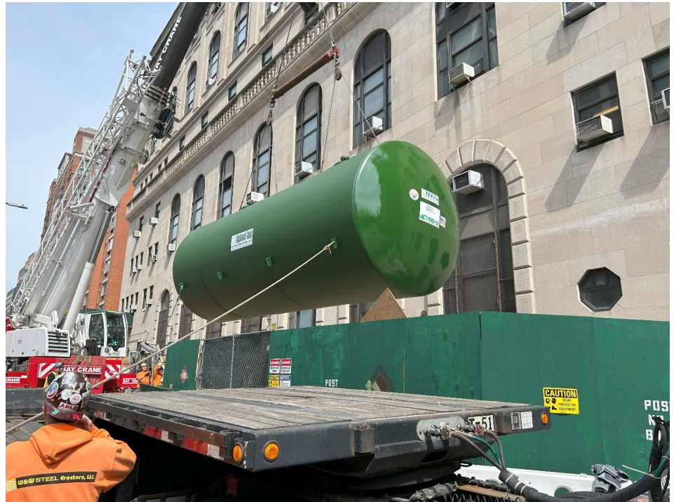
Highland Tank Stormwater Detention Tank
