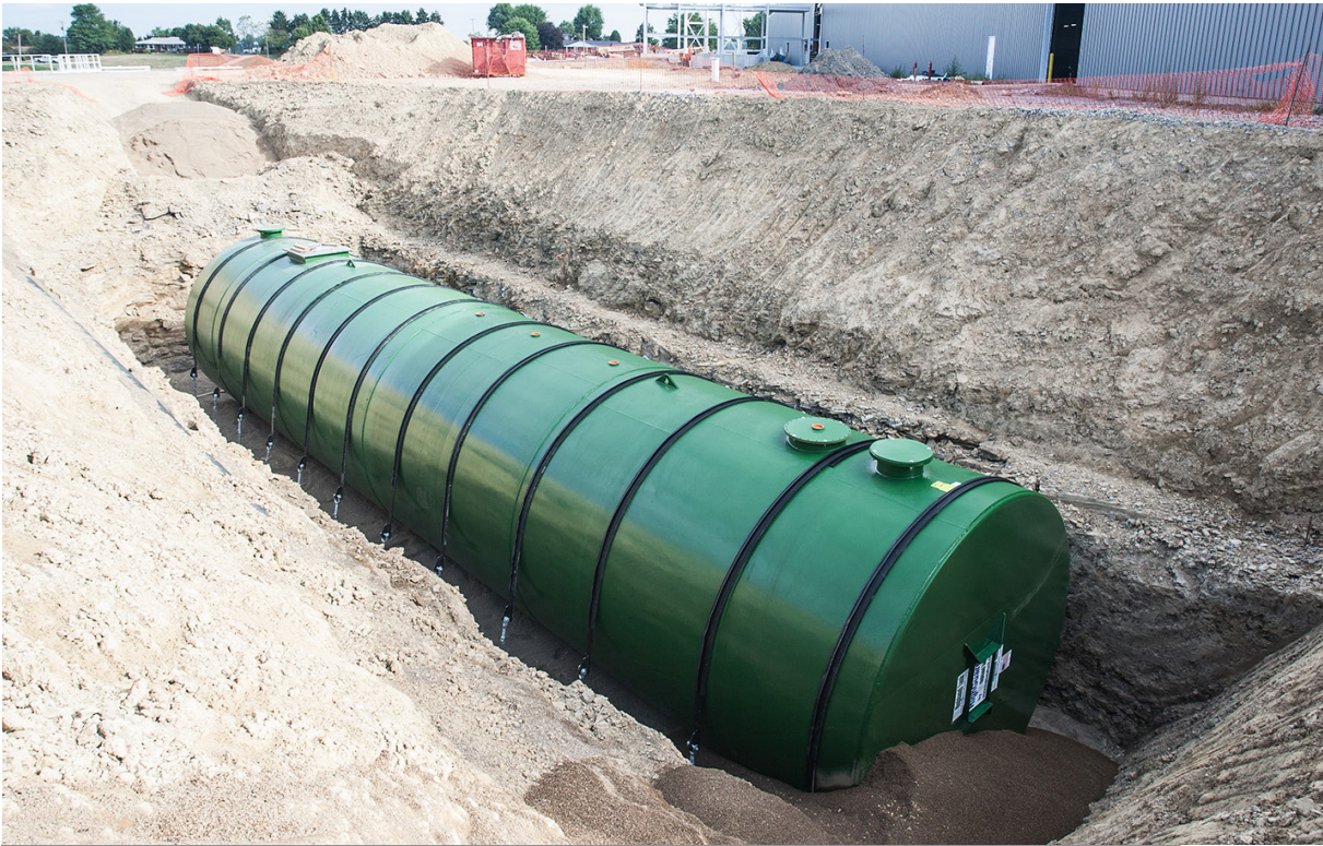
Rainwater Collection Tank
