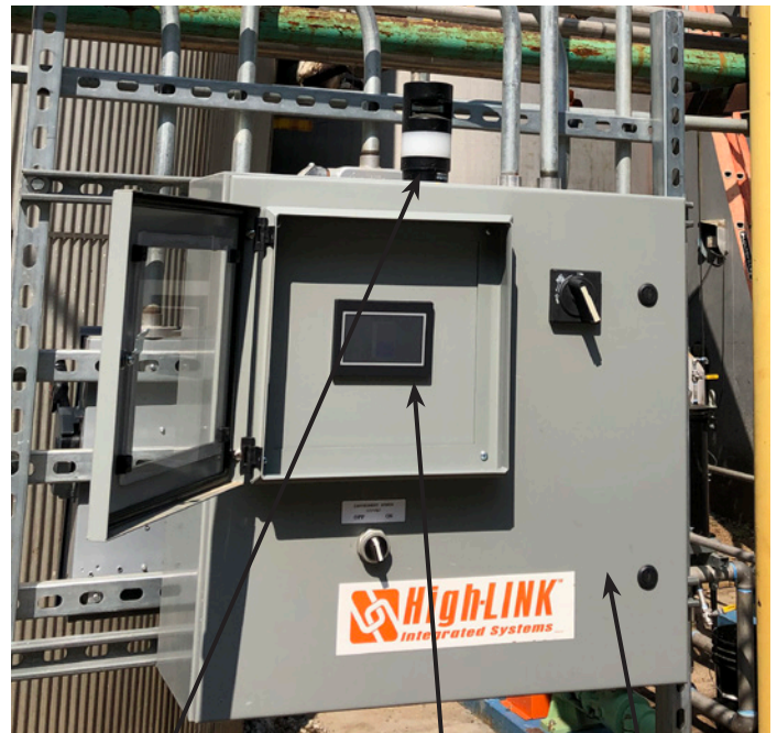
Stack light & siren for alarms
